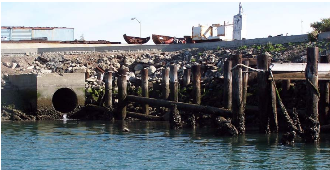
Figure 7-3. Abandoned pilings in San Francisco Bay—romantic reminders of the past or eyesores? (project team photographs)
